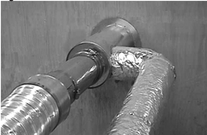
Figure 4 - Inside View of Vent Terminal
