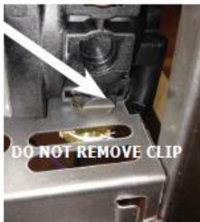
RIGHT SIDE CLIP - INSIDE BOILER JACKET
