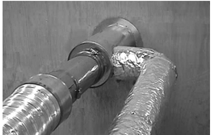
Figure 4 - Inside View of Vent Terminal
