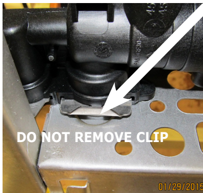
LEFT SIDE CLIP - INSIDE BOILER JACKET
