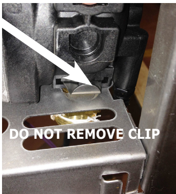
RIGHT SIDE CLIP - INSIDE BOILER JACKET
