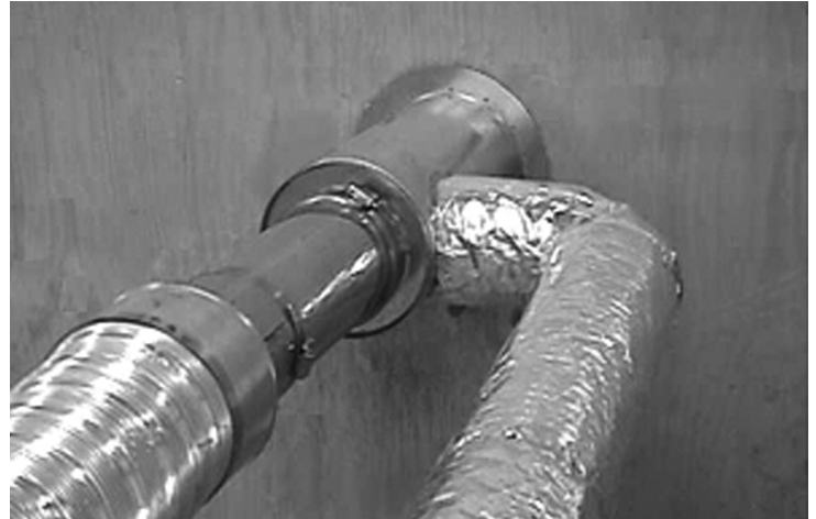
Figure 4 - Inside View of Vent Terminal
