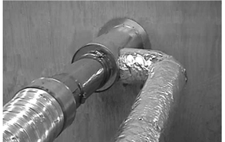
Figure 4 - Inside View of Vent Terminal
